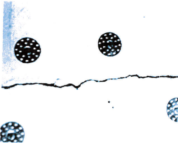
Flat-head wood screws and plaster washers were used to reattach loose ceiling plaster to the wood lath. After the crack is covered with fiberglass mesh tape, all will be skim-coated with a patching compound. Photo: John Obed Curtis.
