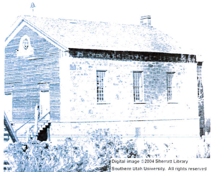
Photo showing the wood siding on the south facade and a stair tower on the north facade. Undated. iropw40. SUU Gerald Sherratt Library
